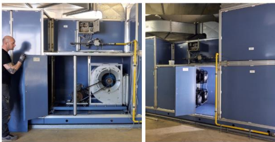
Fig. 2: The old fans were replaced with a FanGrid with three centrifugal fans from the latest RadiPac generation.
