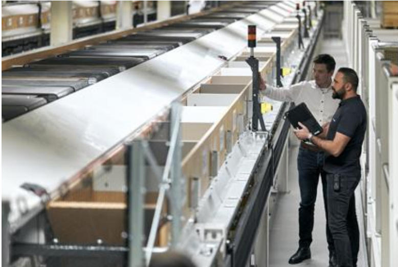
Image 1: The 275-meter-long production facility from the BEUMER Group in the logistics center in Weiden sorts of over 10,000 items per hour.
