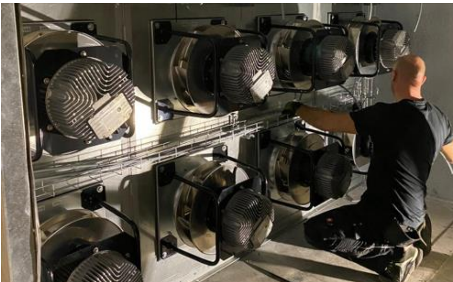
Caption: The Zeithaus automobile museum houses vehicle after vehicle. After a retrofit, the new ventilation system follows suit: one FanGrid houses RadiPac after RadiPac and saves 25 % in energy. (Photo: ebm-papst)
