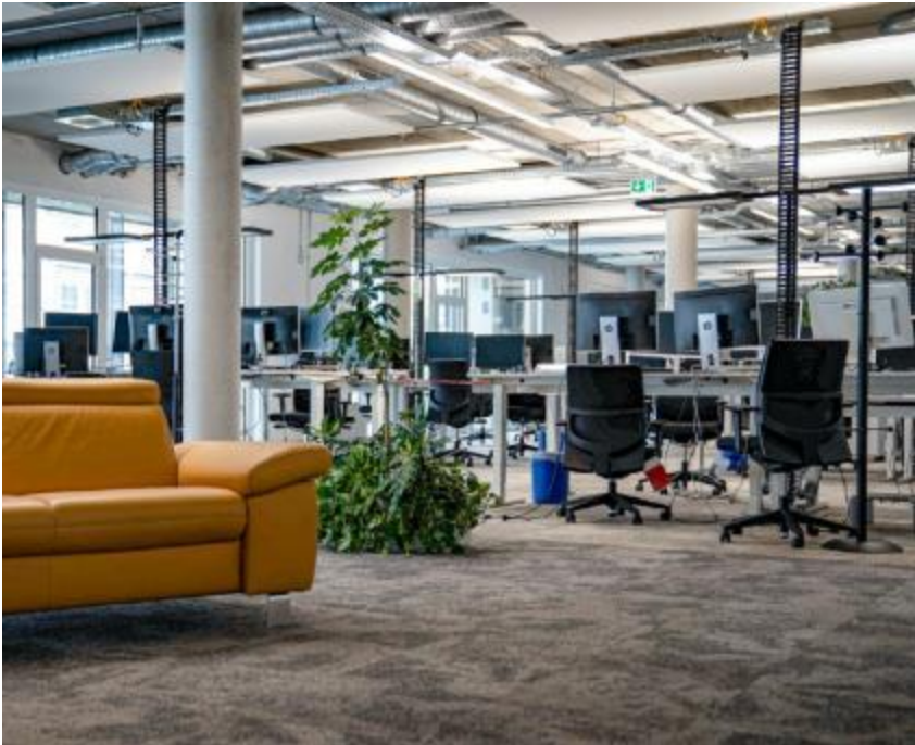
Fig. 1: In Ludwigsburg, one of Europe's first semi-centralized ventilation systems is running with around 300 ebm-papst fans, which supply the modern offices with fresh air.
