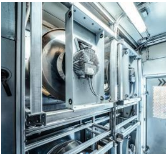
Fig. 2: The new ventilation system with a total of 16 RadiPac EC fans ensures that the dairy products remain fresh at a constant five degrees Celsius.
