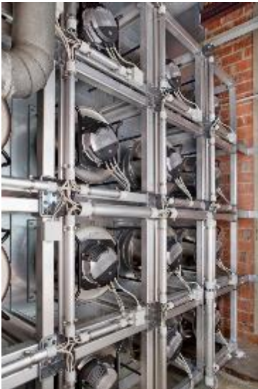
Fig. 1: A FanGrid with 16 centrifugal fans from ebm-papst replaces the defective old fan in the central ventilation system in the Neckarsulm mall near Heilbronn.
