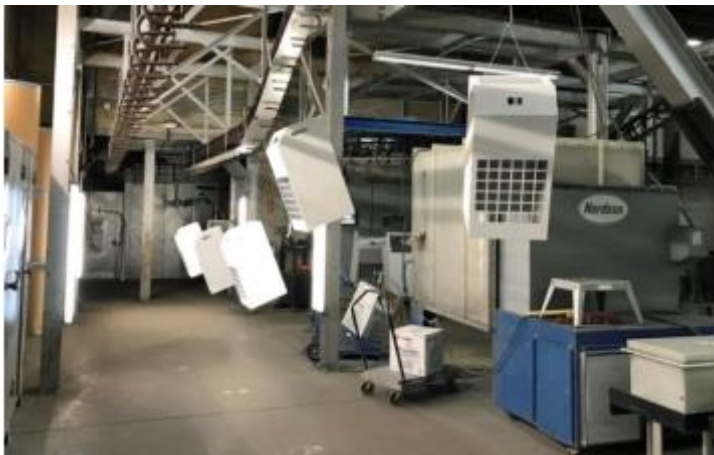
Fig 2: With the help of overtime and weekend work, the first fans together with the metal housings were delivered within two weeks.
