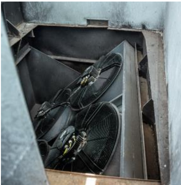
Figure 2: The pivoting metal plate with four fans provides the car deck with energy-saving ventilation.
