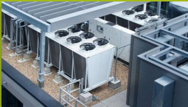
Air Conditioning Technology
