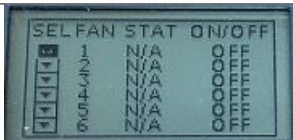
Figure 12: Gateway screen - fan status
